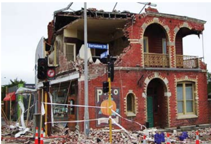
One of thousands of damaged buildings in Christchurch
